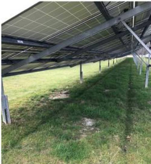
Figure 7: Underside of strings at Partridge Farm solar farm
